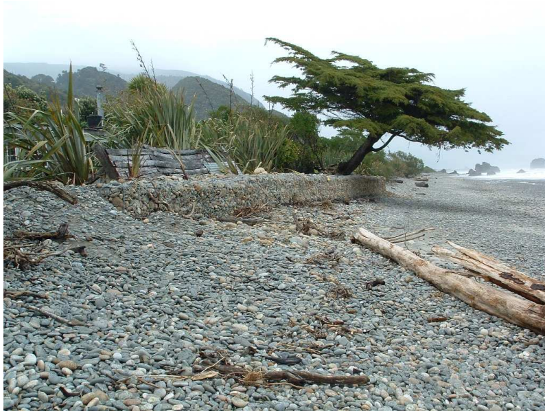
Figure 9: Gabion revetment at 11 Main Road, Ngakawau. The wall is not aligned with the coastline and is likely to suffer outflanking at the southern end. Also by not maintaining the upper gravel beach in front of the defence also makes it more prone to damage and undermining and less effective in preventing overtopping.
