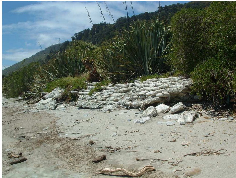
Figure 13: Concrete filled bag revetment at 31 Main Road Hector. This shows the results of an inadequate construction including inappropriate construction material, lack of proper foundation, underlayer and end design. This wall is unlikely to survive much longer.
