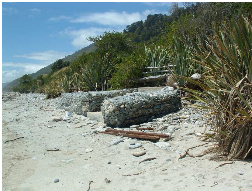
Figure 14: Gabion wall at 35 Main Road Hector. The wall has been built over the upper beach making it more prone to damage and outflanking.
