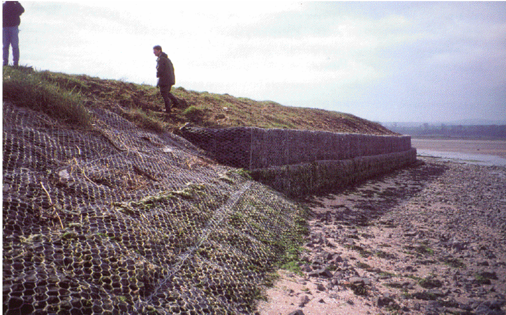
Figure 6: Example of a sloping gabion revetment which tends to have less impact and are more stable than a vertically constructed gabion wall. Blown sand (e.g., along the Hector frontage) is also able to accumulate on such revetments, softening their appearance (Photo: Scottish Natural Heritage, 2000).
